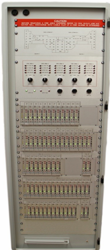
Multi Zone LHDC control panel, complete with sprinkler control Panel and mimic diagram. Construction: Floor standing 19" cabinet with swing frame and glazed door. Application: Nuclear Power Station – Cable Flat Protection
