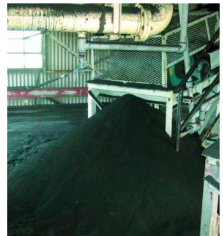
Coal accumulation at a conveyor tail
