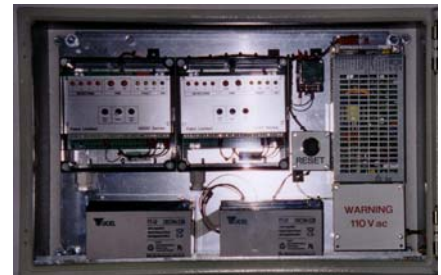
Typical Control Equipment Series 5000 Monitors and PSU Patol Limited - Reading UK
